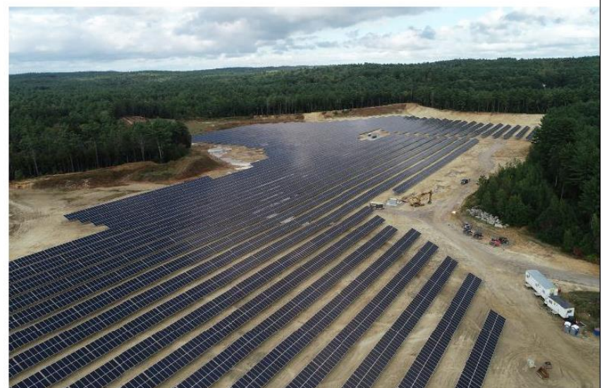
[Happy Hollow Community Solar(PV 7.1MW, ESS 3.3MW)]
