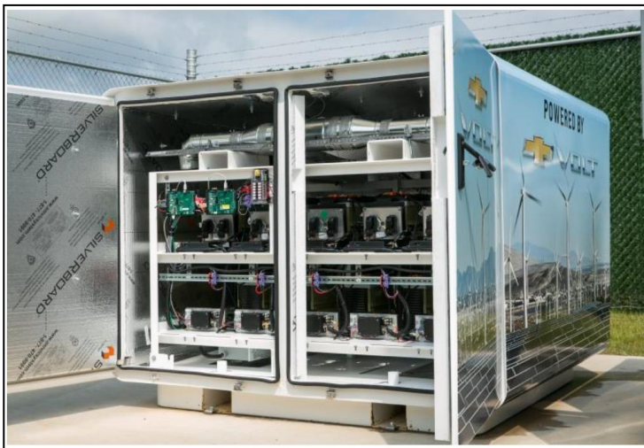
Energy Storage GM Volt Batteries Milford, Michigan
